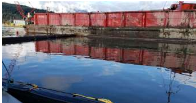
Continued use of silt curtain and sealed scow for dredging and transferring to dedicated disposal site in new containment facility (west berm).
