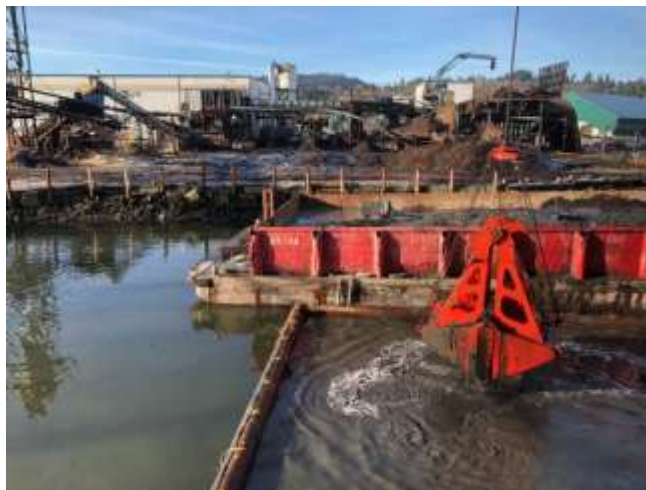
Remedial dredge at Flavelle Cedar sawmill: Envirobucket, silt curtain and sealed scow. Recovered material sent for upland disposal.
