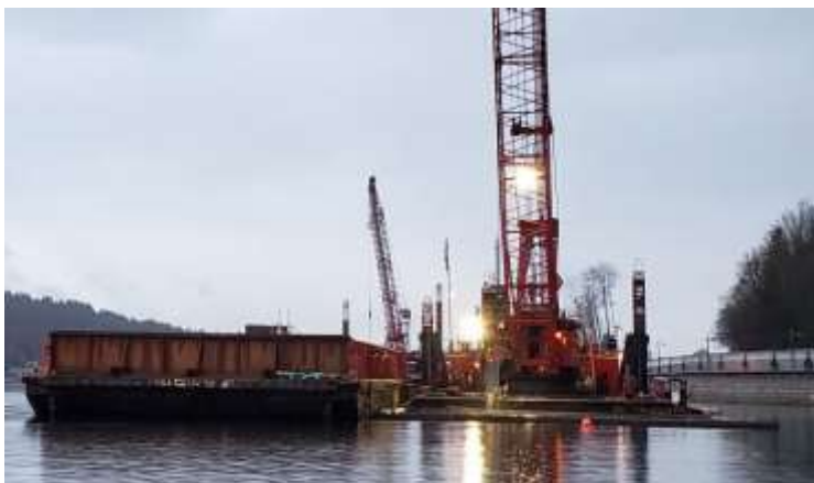
PAH remedial sediment dredging near Reed Point Marina with silt curtain frame and sealed scow.
