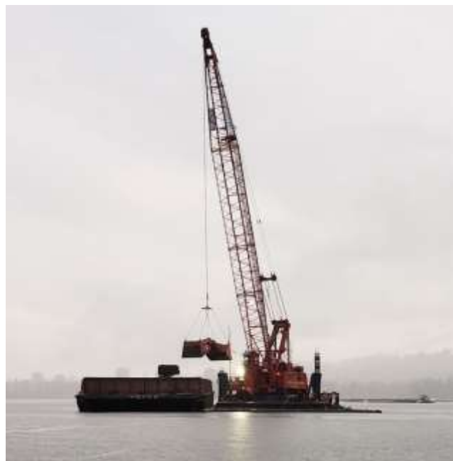
PAH remedial dredge disposal at designated location in new containment facility (west berm) using Envirobucket, silt curtain, suitable duty cycle and sealed scow.
