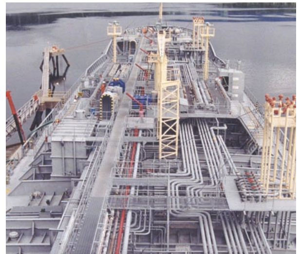
Liquid Tanker from above: the Matsukaze's tanks and manifold compartments.
